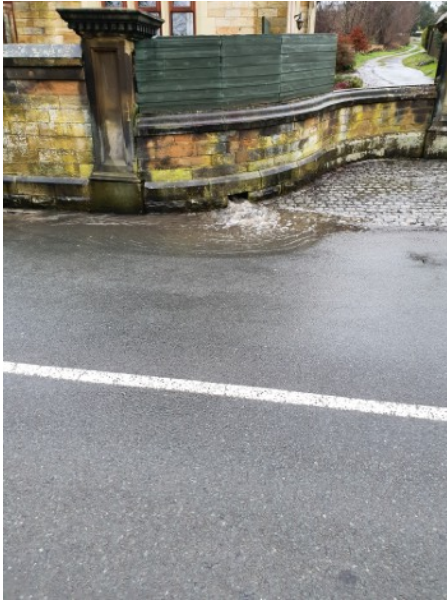
Photo: water pooling outside Oakland's Lodge
